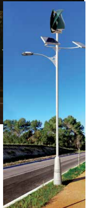
The innovative Eolgreen hybrid street lighting system is turning Mount Roskill's Jasper Avenue car park
